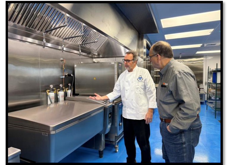
Existing Building Electrification
